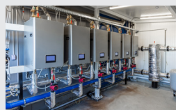
Mechanical Equipment Connections
